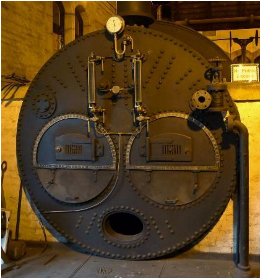
Figure 38. One of the two Lancashire boilers installed in 1902. Although these bear the name of Teasdale Brothers of Darlington, their construction was in part down to Goodfellows of Manchester, with Teasdale Bros. acting as a main contractor for the new beam engine and associated works of 1900-04
